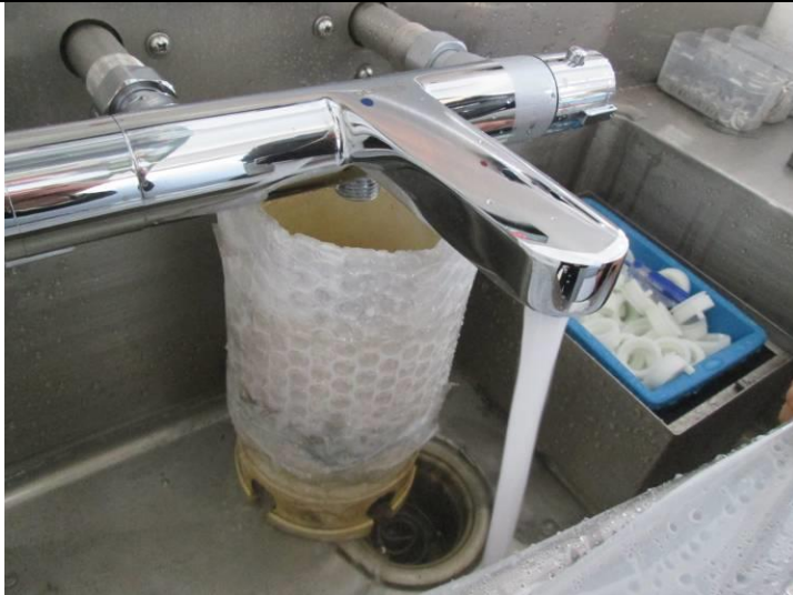
Check the unit to keep the flow of water by the aerator
